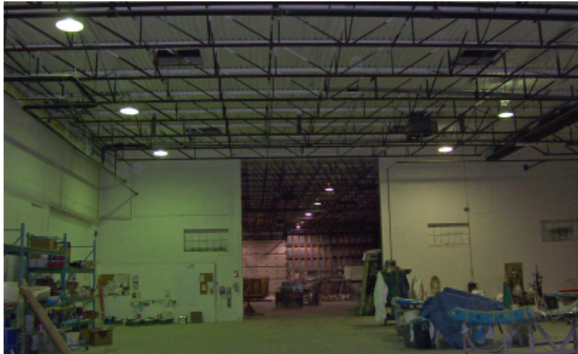
BEFORE: Five of the highbay lights that were replaced can be seen in the photo. Note the greenish cast to the lighting which is characteristic of Mercury vapour lights.
